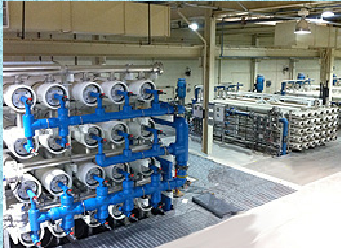
City of Scottsdale's Water Campus - Comparison of 2.4 MGD train (left), 1 MGD trains (right) with 8-inch elements. (WDR September 10, 2012)
